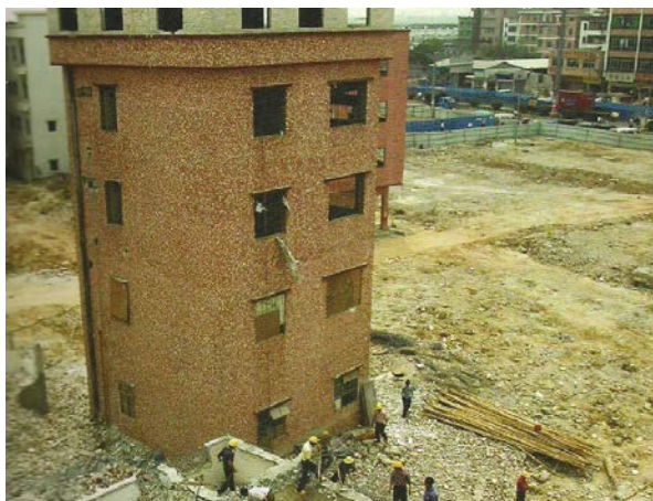
Figure 1. A "nail building" in VIC in the middle of a demolition process. Source: Ai, S. A. (2014). Villages in the City. A Guide to South China's Informal Settlements. Hong Kong: Hong Kong University Press.
